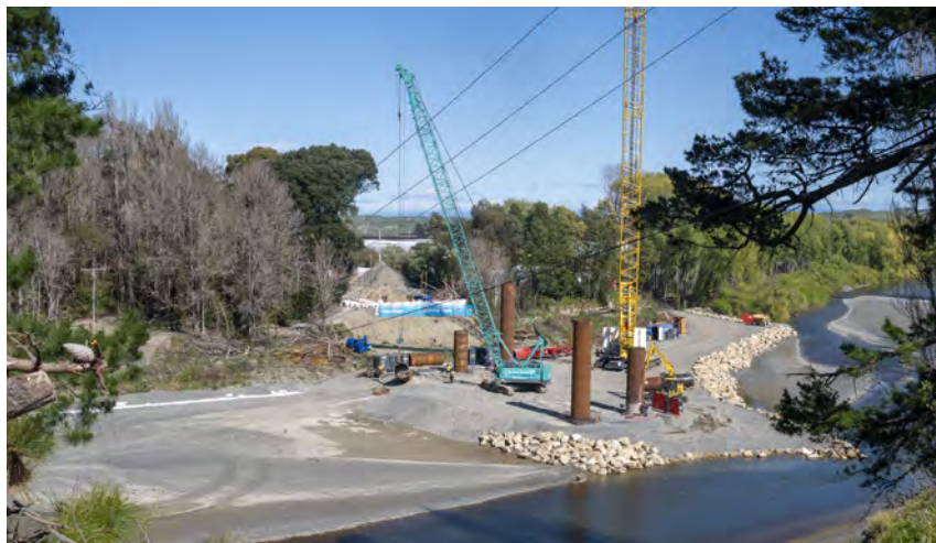
Bridge piers being built for the replacement Puketapu Bridge on the Tūtaekuri River. The original bridge was destroyed during Cyclone Gabrielle. The replacement bridge has a more resilient design using modern construction standards.
