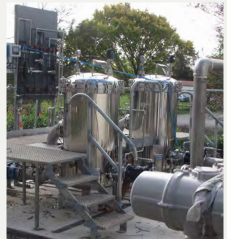
ELABORATE WATER TREATMENT FOR HAVELOCK BORE 3
