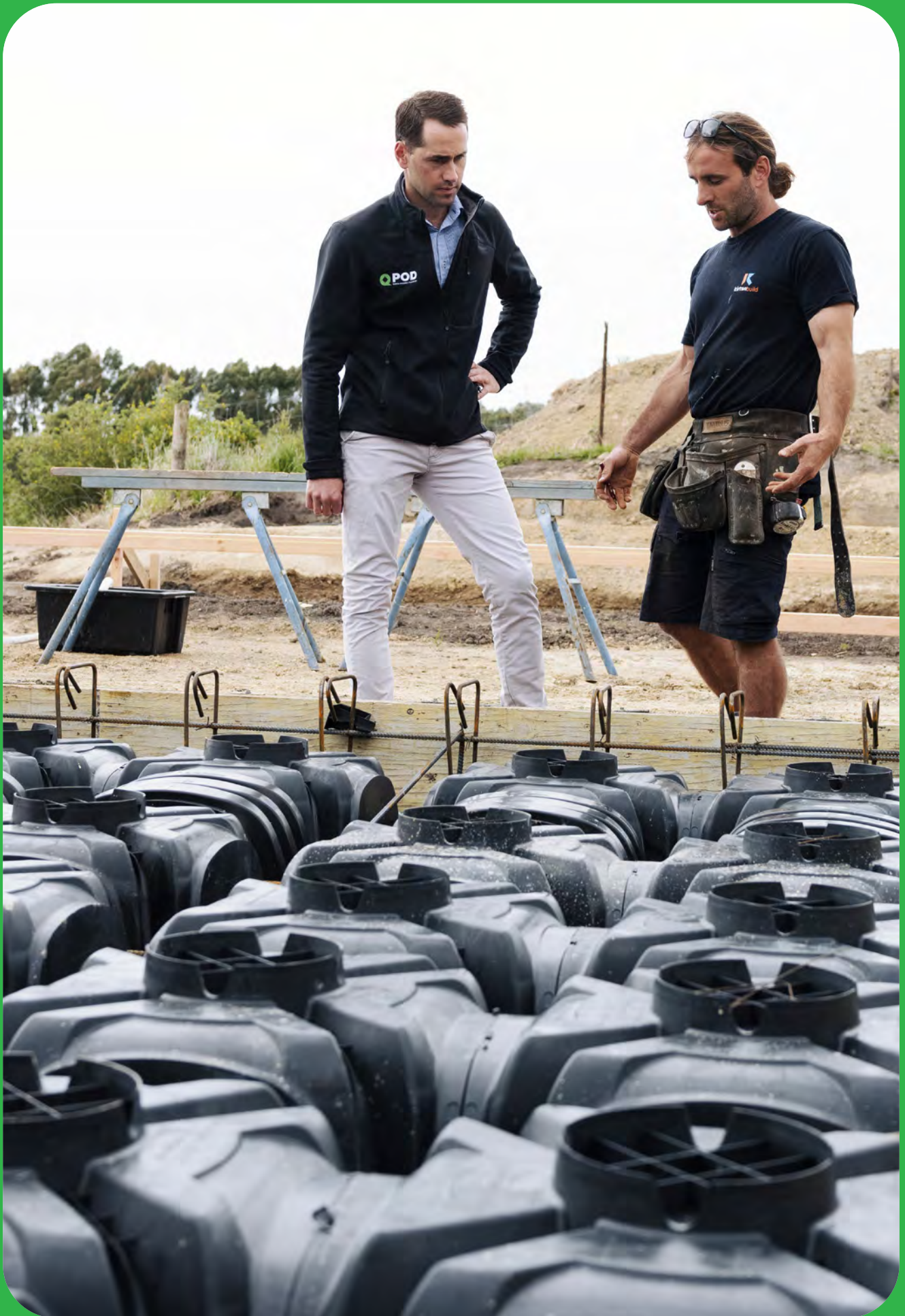
Peter Crawshaw and builder Bernie Kirton installing Qpod recycled plastic floor insulation.
