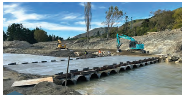
The Ellis-Wallace low-level crossing. Photo: Quality Pumping
