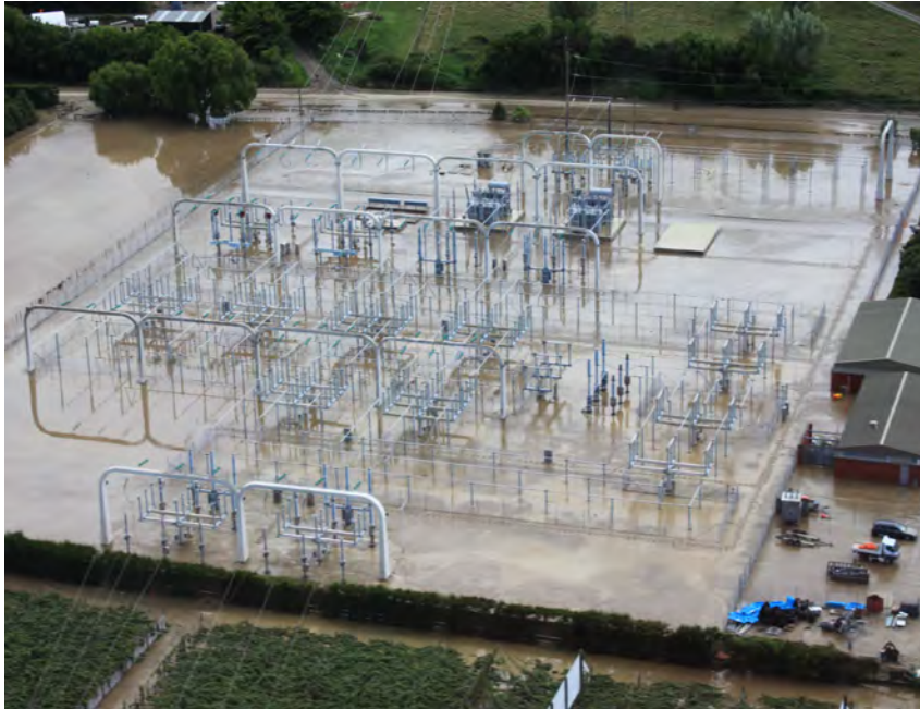
Redclyffe substation under water.
